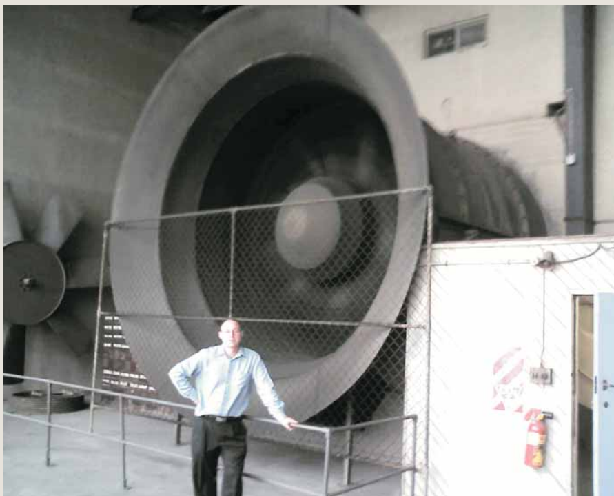
One of the fresh air intake fans installed at the Lyttleton Road Tunnel
