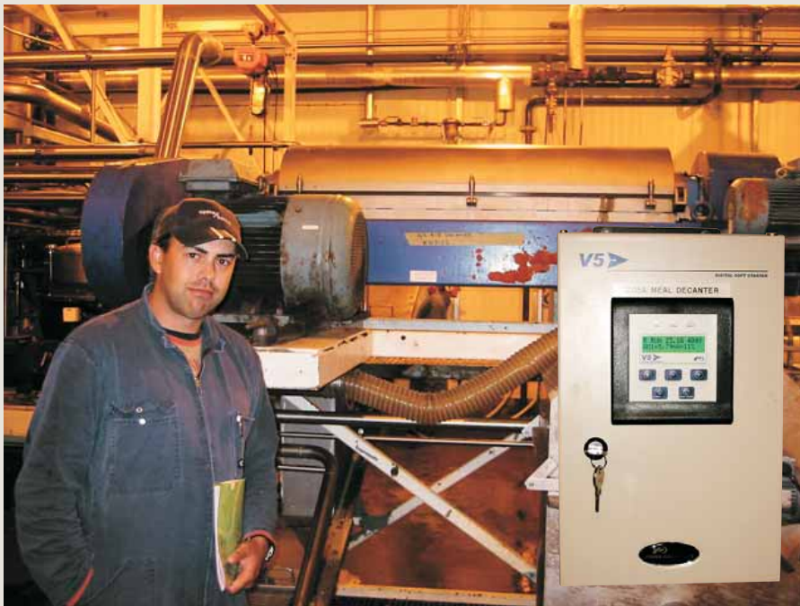
Corey Brett, SPM Engineering Manager, with the 22kW Decanter and V5 Soft Starter (inset).
